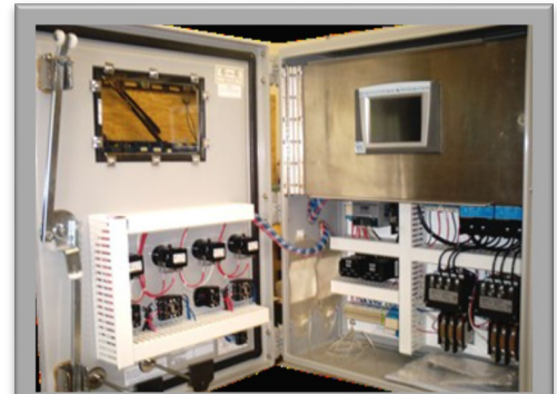
Simplex Pump Control Panel
