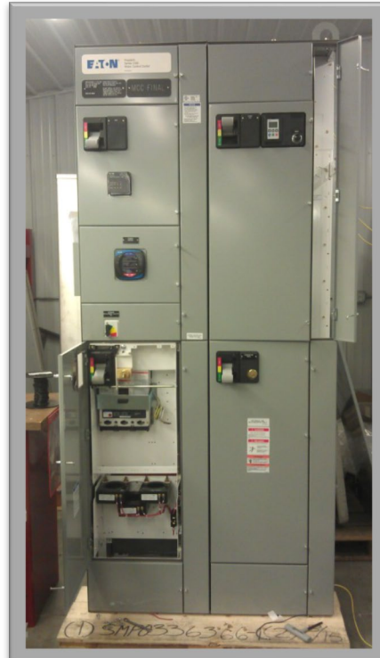
MCC Power Panels
