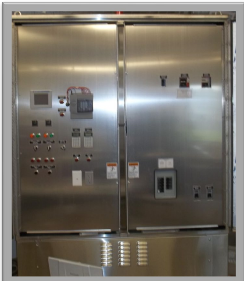
Triplex Pump Control Panel
