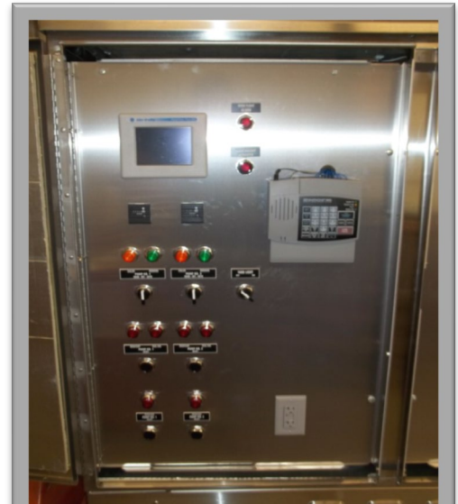
Duplex Pump Control Panel
