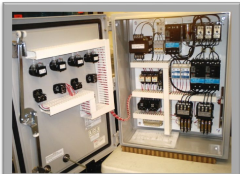
Clarifier Control Panel
